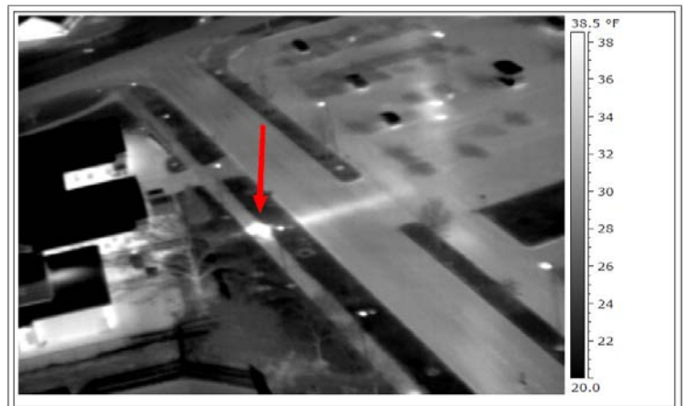
Cornell uses infrared images to help prioritize steam line insulation repairs. Lighter areas in the above image reveal heat loss from the “Guterman Line” steam piping.
